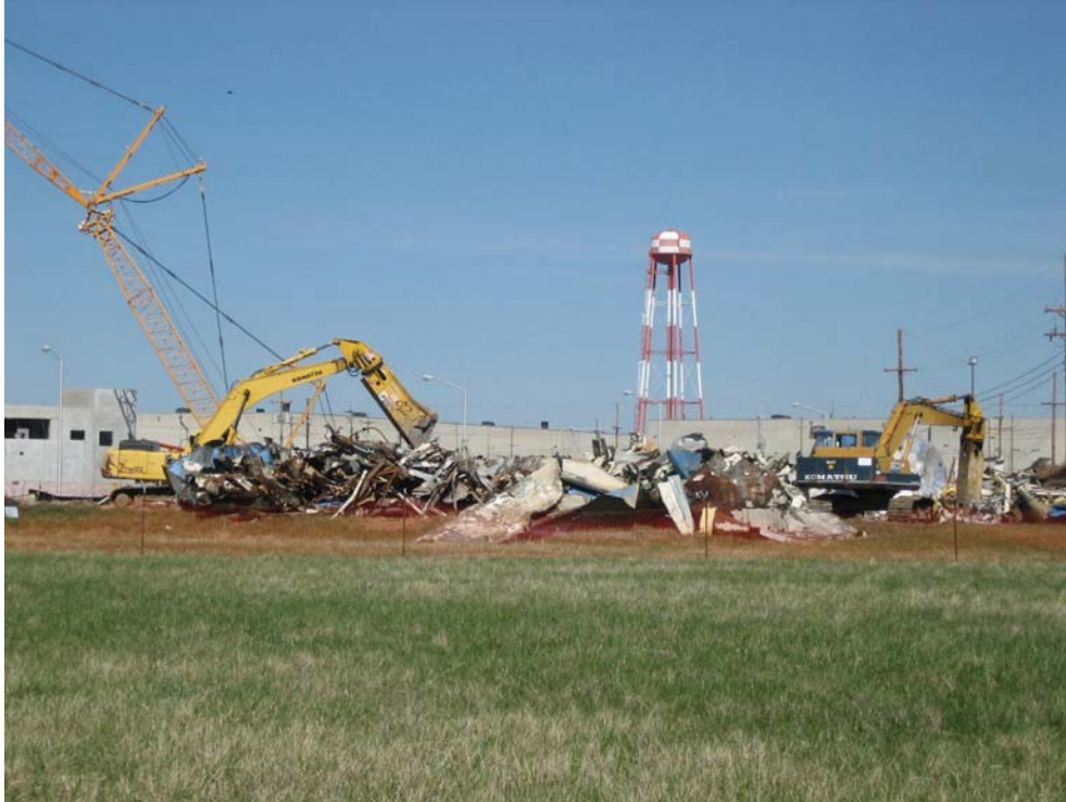
Pictured at left is the X-616 Liquid Effluent Control Facility nearing completion of demolition activities.
