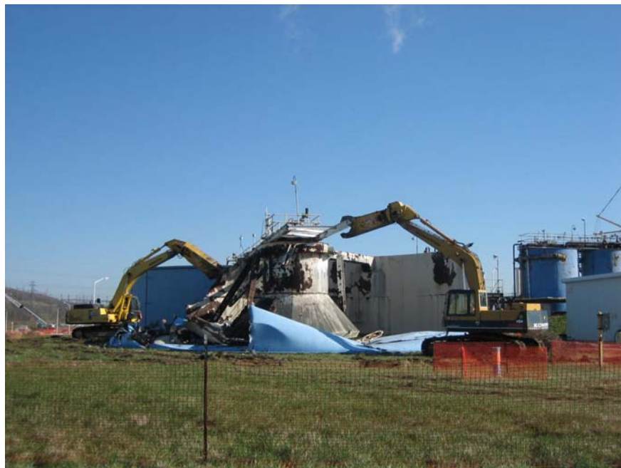
Demolition of the X-616 Liquid Effluent Control Facility started April 4 and was completed by mid-April 2006.
