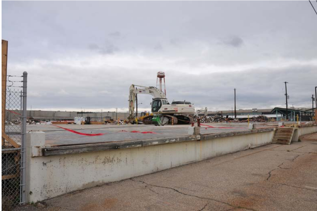
Demolition of the Shipping and Receiving Building structure was completed September 25, 2009 at the Portsmouth Gaseous Diffusion Plant
