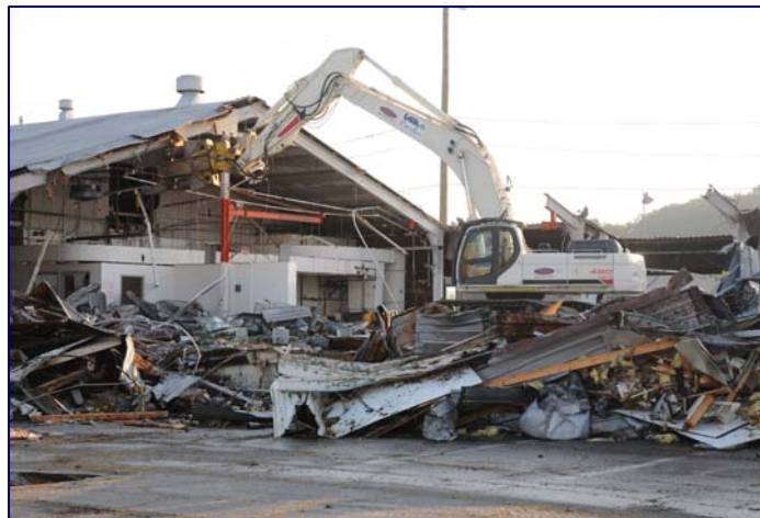
Demolition of the former Shipping and Receiving Building at the Piketon plant site in September 2009
