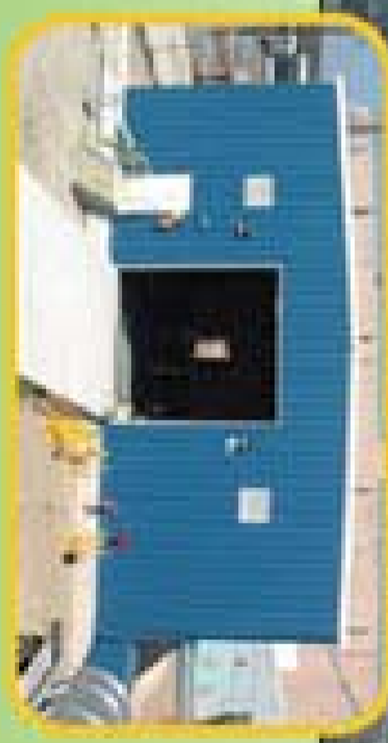
One of four groundwater treatment facilities that treat 26M gallons/year from 5 plume areas
