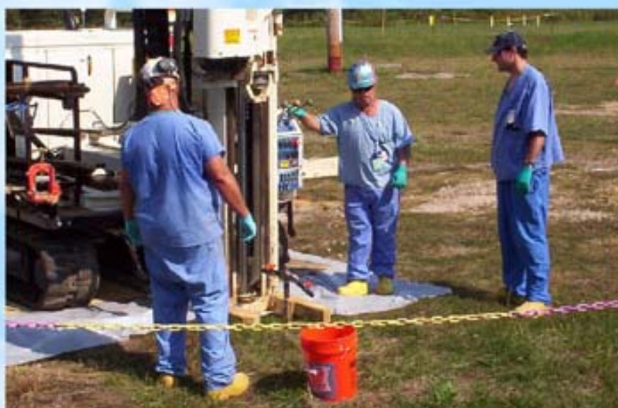
Chemical oxidant injection treatment of a groundwater plume with concentrations of TCE was effective in treating the upper soil layers. Additional cleanup actions will be taken to remove the source area of the groundwater plume.
